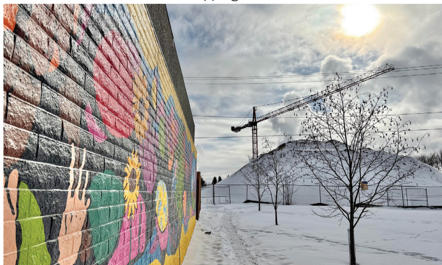
Crane over future senior complex, seen from the mural in the pocket park.
